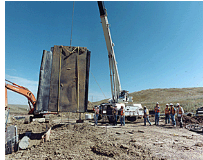
Installation of the high-density polyethylene panels at the East Trenches PRB project at Rocky Flats.
